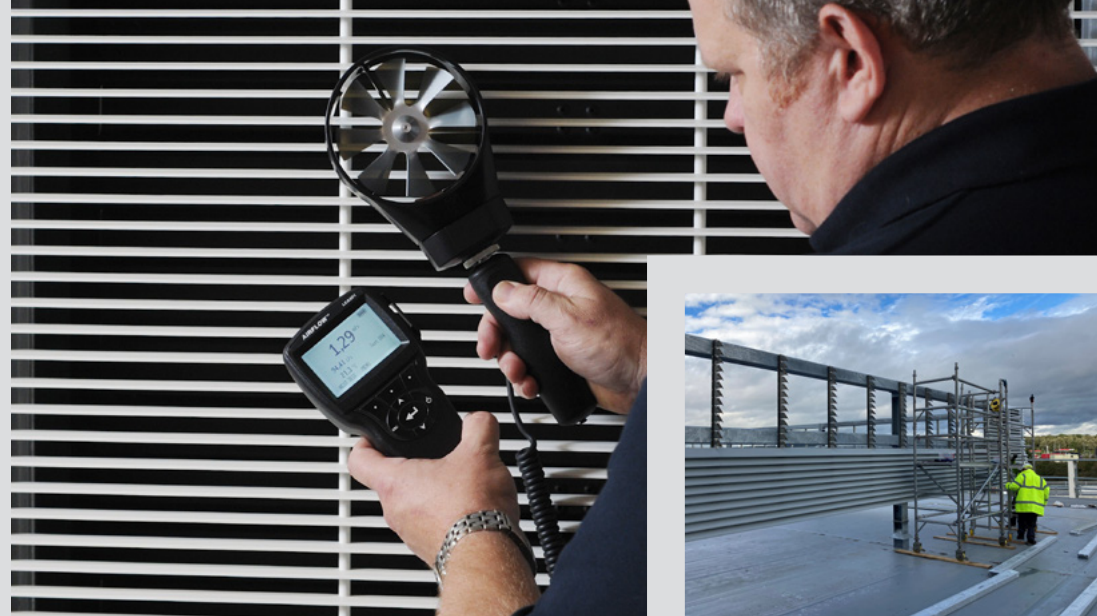
Above: Checking airflow on installed louvre panel. Right: Installation of 1UL/DH louvre.
